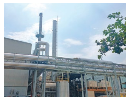
Waste Heat Recovery Unit
